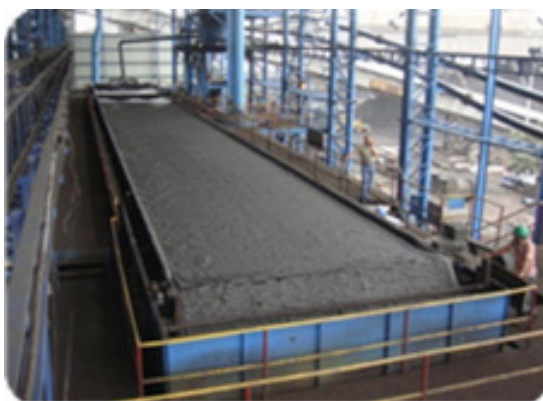
145m 2 Delkor Belt Filter installation at Washery III West Bokaro Tata Steel
