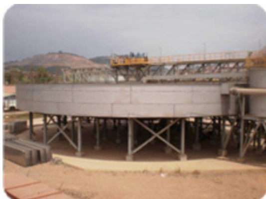
35m Clarifier ready for operation
